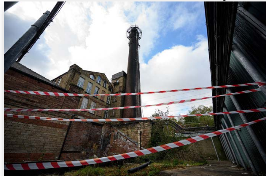
Damaged cabling and telecommunications equipment following a fire at a phone mast attached to a northern England, on April 17, 2020.
