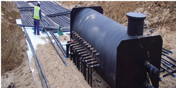
Edgerton Hospital and Health Services geothermal system.
